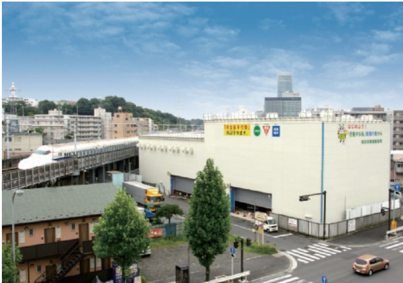
泥水シールド工事防音対策 Measures against noises produced by the construction of mud water shields
